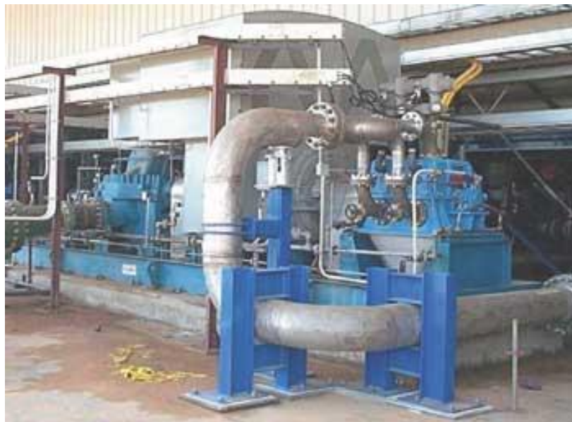
Figure 2-2: The Trinidad SWRO Plant Implementing Francis Turbine
