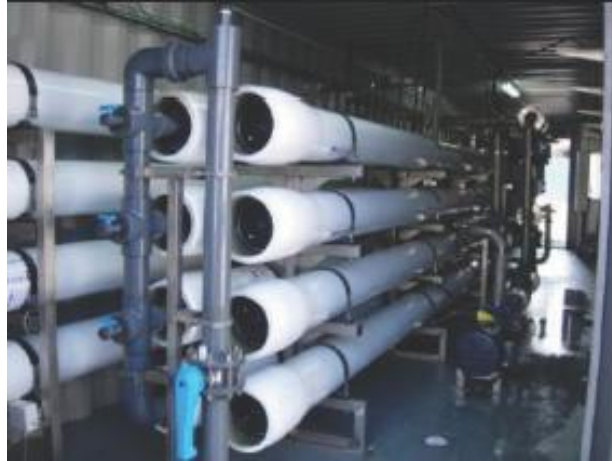
Figure 8-8: Desalitech CCD™ Unit
